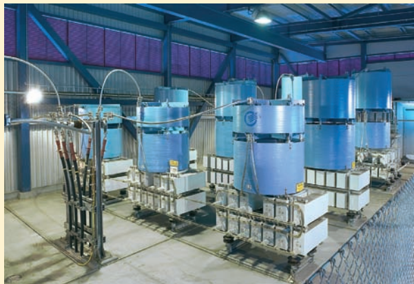
■ FIGURE 11.19 A compensation capacitor installation. (Courtesy of Nokian Capacitors Ltd.)
